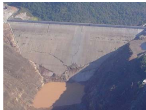
Fracture lines are evident in the concrete face of the Campos Novos dam. (Photo courtesy Friends of the Earth)
